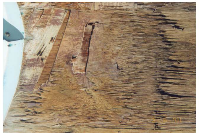
This plywood fan deck has rotted away making it dangerous for workers to walk on.
