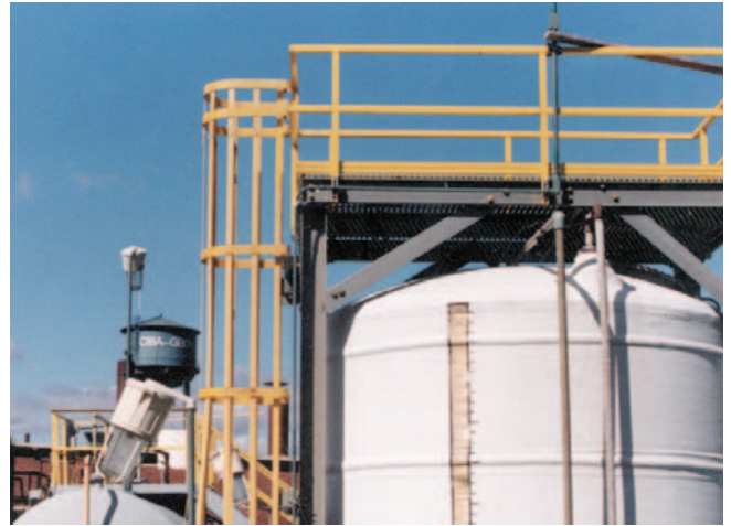
This fiberglass ladder and ladder cage provide worker access to a maintenance platform at a Ciba Geigy plant in the northeastern United States.
