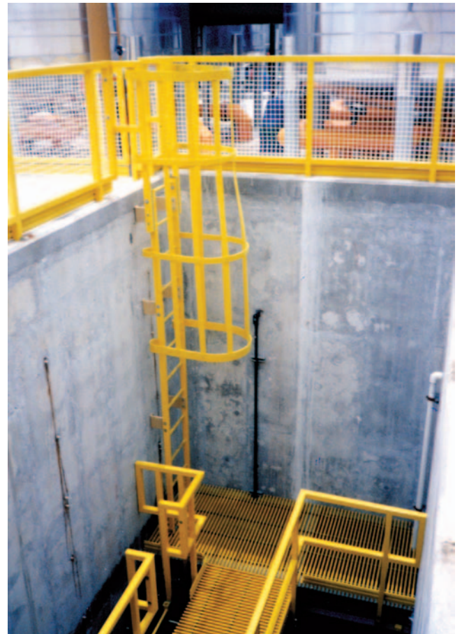
Fiberglass access ladders are used throughout the service areas of Sea World, Orlando, FL to resist saltwater corrosion and reduce maintenance
